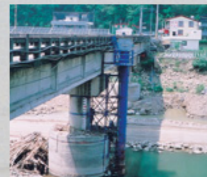
▲Bian Bridge Buoy Water level Tower
