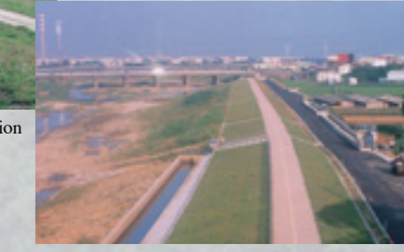
▲The Right bank landscape restoration Construction Project of Railway up to Tai 1 Rd. Bridge in Fongshan River.
